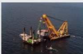
Asian Hercules II provided heavy lift assistance during the construction of the world's largest offshore windfarm off Danish Coast
