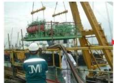
▶ Process module for the World's largest FPSO Conversion Project "BW Enterprise" with a production capacity of 600,000 BPD.
